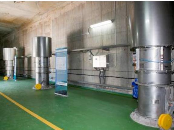
Turbine room of Mutriku OWC, Basque Region Source: EVE
